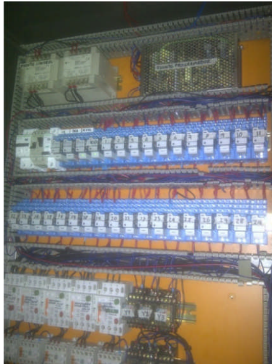
Figura 5: Tablero de control Jigger
