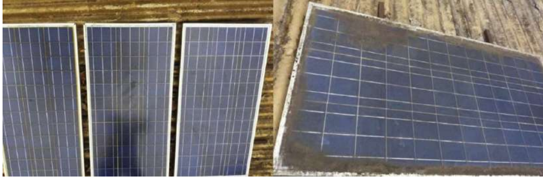
Figure 1.5: PV panel degraded due to exposure time. Adapted from: [20]
