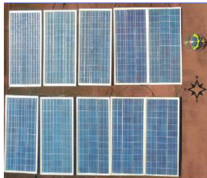
Figure A.43: PV system and proposed prototype installed at 6^{\circ}14'39.9''N - 75^{\circ}33'07.0''W .
